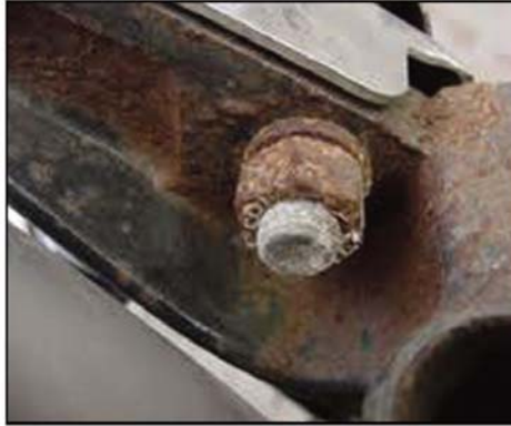
Figure 11. Rusty Bolts can cause PIM.
