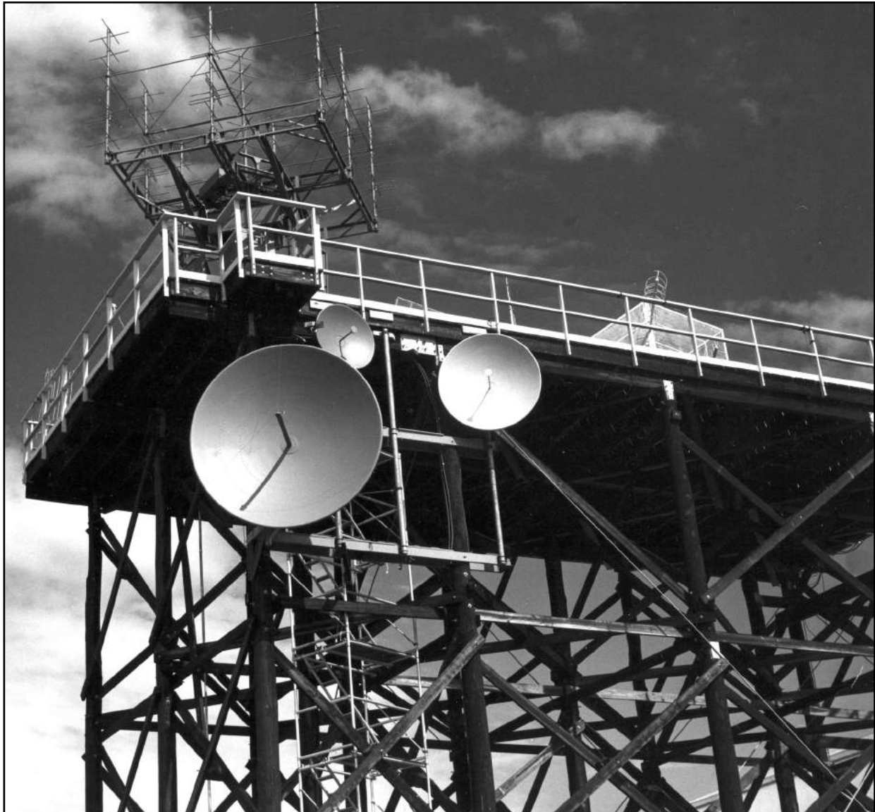
Photo 28-4.2. NASA platform at Cape Canaveral supporting antennas communicating with various spacecraft on launch pads during pre-launch operations. The two dish antennas were used for communicating with the RELAY spacecraft. The small dish is the 4.17-GHz downlink antenna, while the large dish is the uplink antenna. The dish antennas were engineered by the author.
