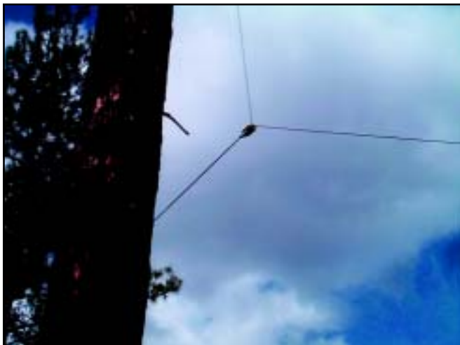
One of the tree supports and insulators. I’m using high-voltage electric fence insulators here. The tie down rope passes through a big screw-eye screwed into the tree.
